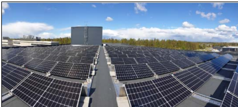
Solar Panels at plant in Sweden
